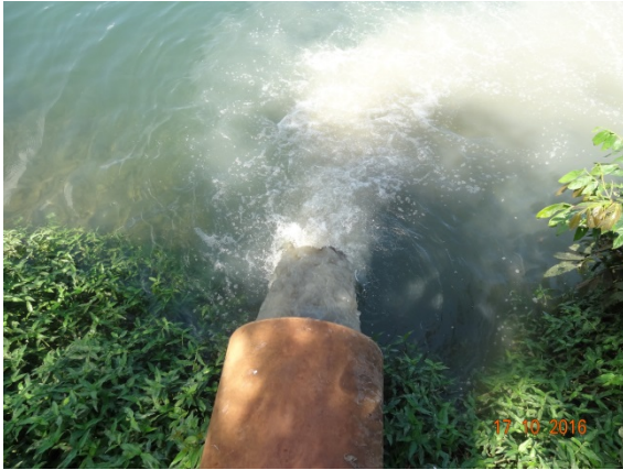
Foto 1 – By pass da EEE IV (17/10/2016)
